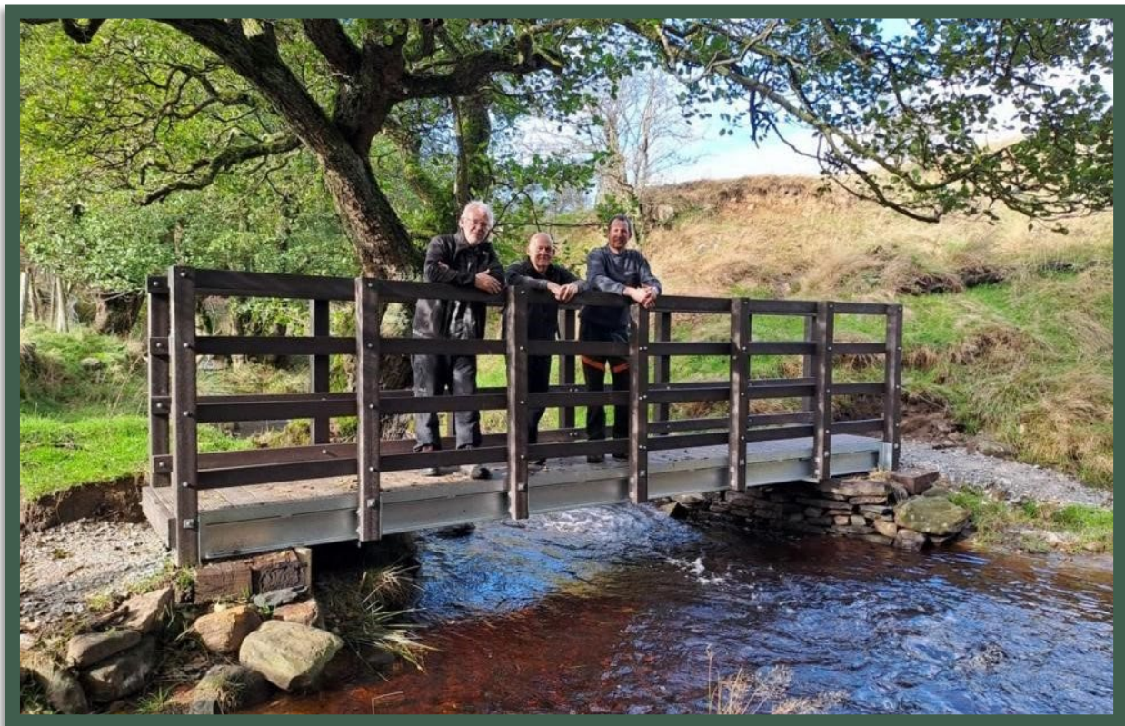
Image 8 | Rick Hill (Countryside Officer, Bradford Council), Nigel Howe (Bridges Officer, PNFS), Max Kopasz (Countryside Supervisor, Bradford Council) on a newly erected bridge across Slippery Ford Beck, Keighley FP29. (Image: Bradford Council)
