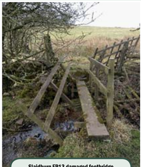
Slaidburn FP13 damaged footbridge
