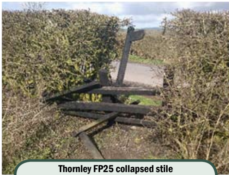
Thornley FP25 collapsed stile - easy to walk over!
